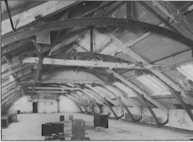
The main attic of Beehive Mill, showing the unusual cast-iron and timber truss construction.
