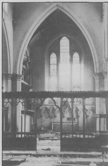
Christ Church, Heaton Norris, 1977. Vandalism in the redundant church. Peter Pownall, A Bramhall Farmer, 1765-1858 — a transcript with an extensive glossary, was published. (Still available, price £4.95). More material is being collected and work is continuing slowly for both Bramhall and Hazel Grove.
