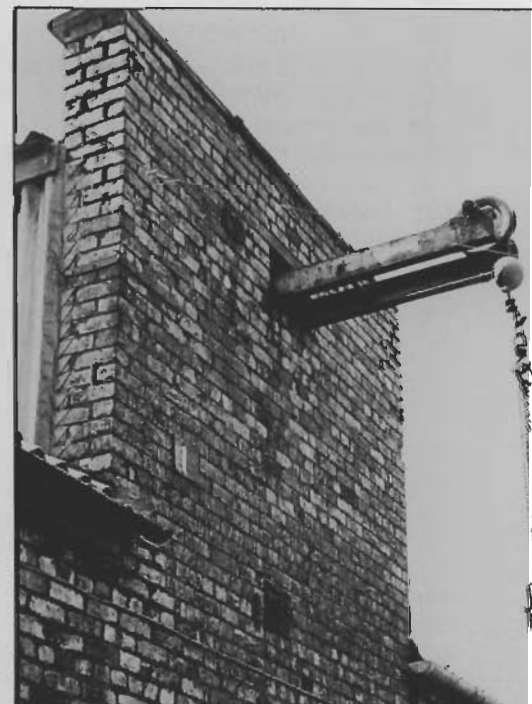
Hoist. Detail from rear of Peel, Williams & Peel.
